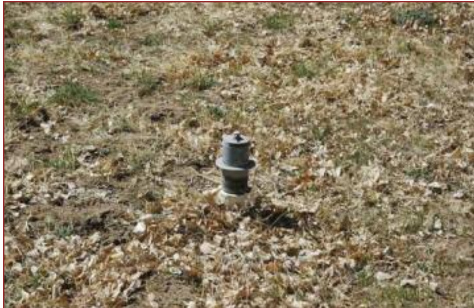
Pop Up Irrigation Sprinkler
